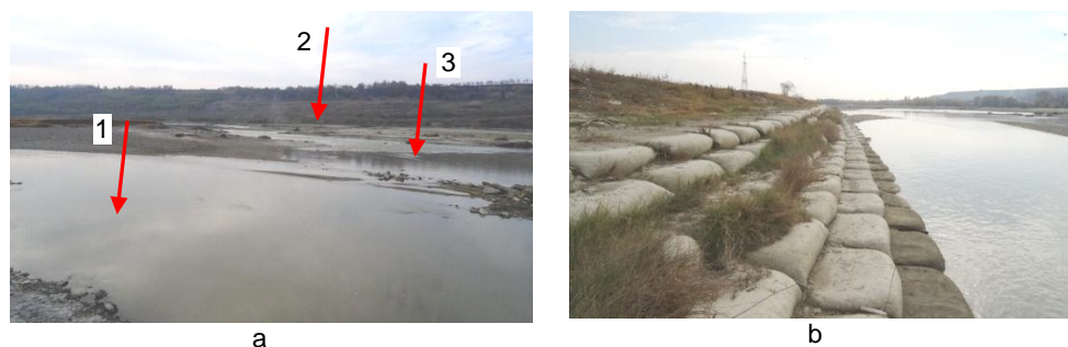
Fig. 3 The state of the natural site in the Pildești area on the Moldova river: a - the riverbed branching zone (year 2015), 1 - the new bed in the capture area, 2 - the old riverbed, 3 - digging dam; b - view of calibrated bed and shore defence in capture area (year 2018).
